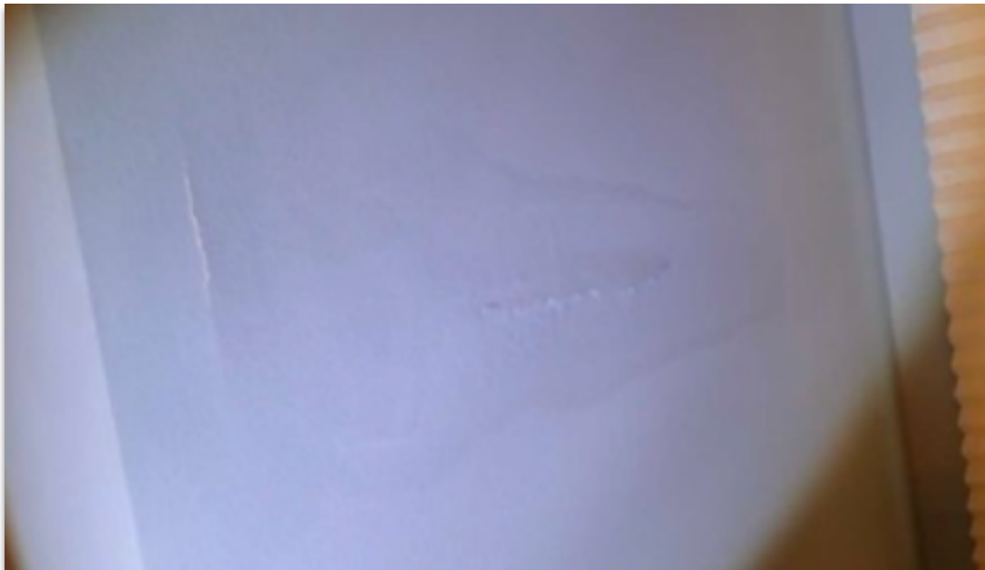
Photo 18: Interior water stains
