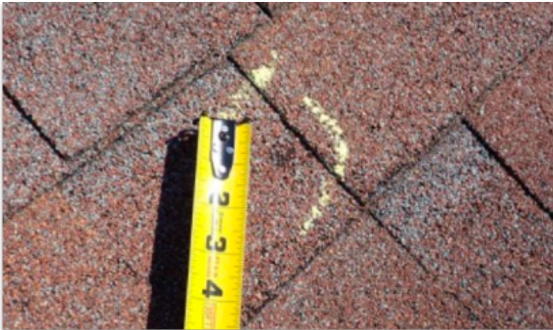
Photo 9: Damage close-up photo
