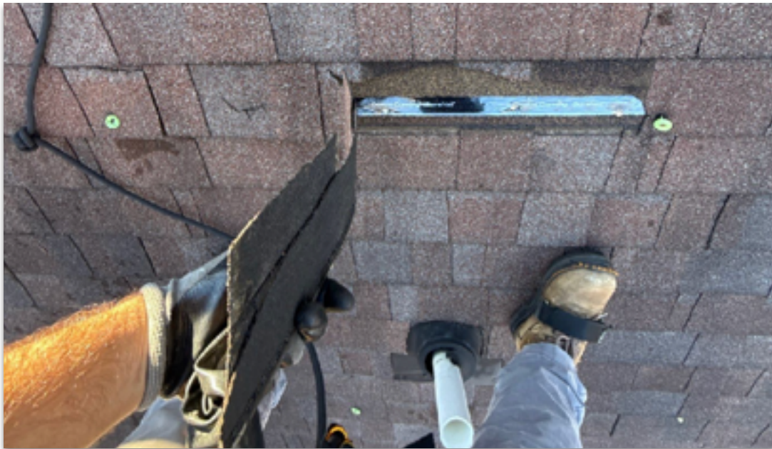
Photo 20: Torn shingles on back of home
