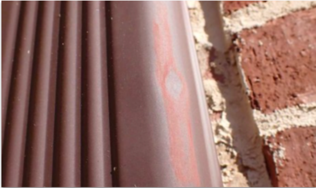
Photo 15: Dent to gutter
