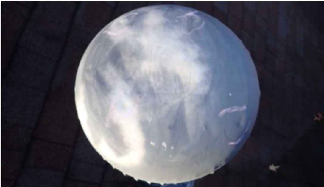
Photo 16: Dents in vent on roof
