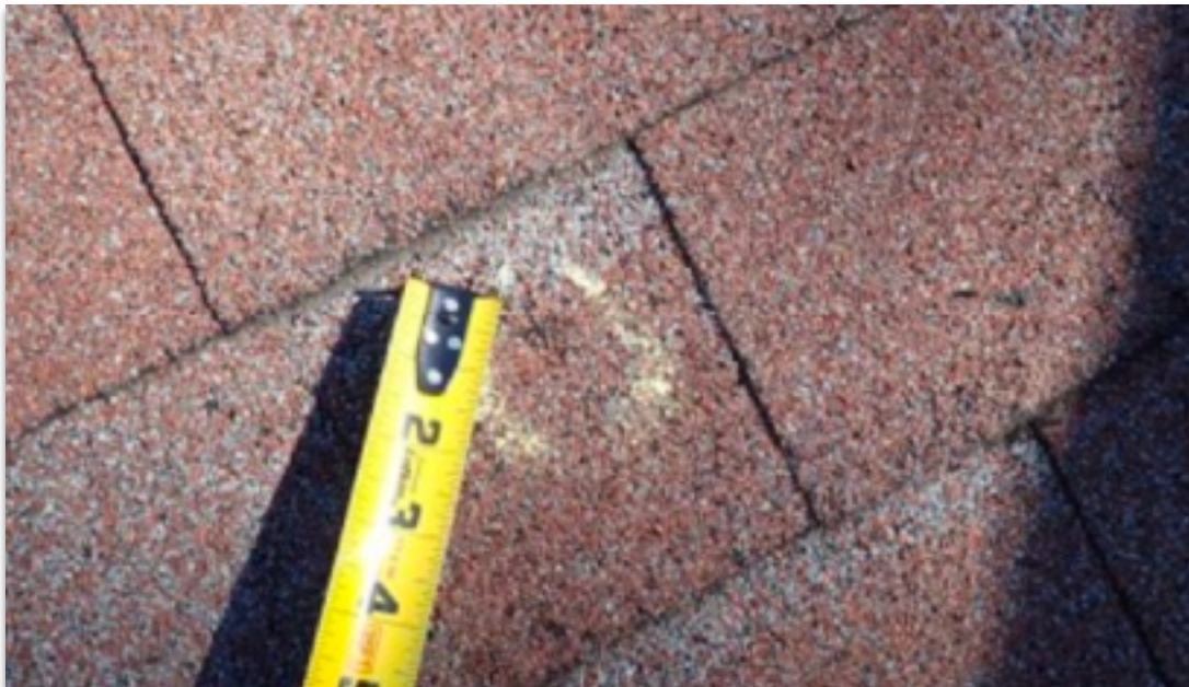
Photo 8: Damage close-up photo
