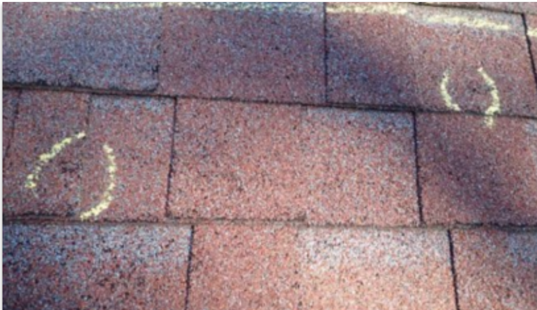
Photo 10: Damage close-up photo
