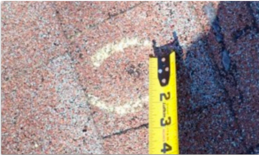
Photo 7: Damage close-up photo
