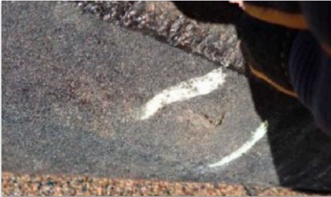
Photo 5: Fracture on back of shingle
