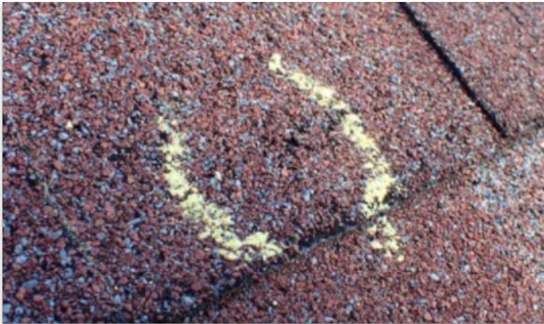
Photo 11: Damage close-up photo
