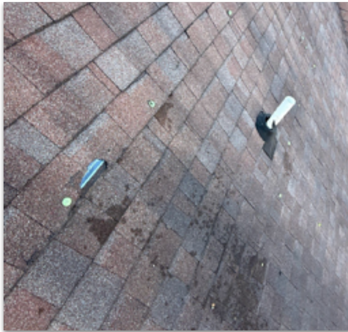
Photo 19: Damaged shingles on back of home
