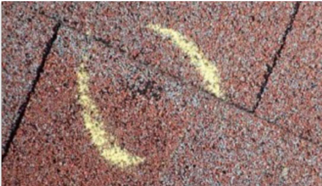
Photo 12: Damage close-up photo
